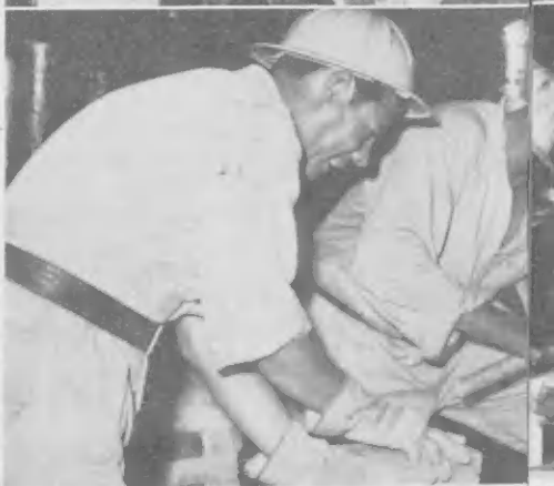
WORKERS START ripping out the furnace convection section. The rope prevents the workers from falling. Workmen, below, clean firebrick which can be reused on the new furnace. A suspended bridge-type wall is being built.
